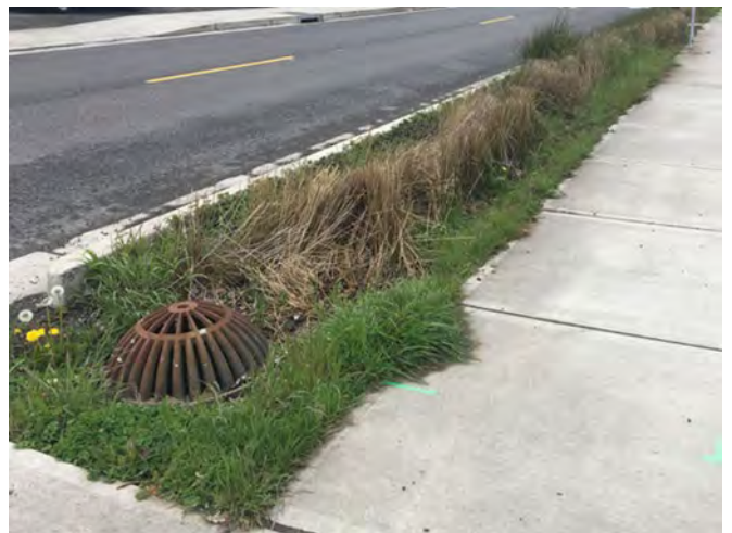
Above ~ Street-level Stormwater Planter
